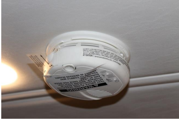
Typical Smoke & CO monitor combination monitor
