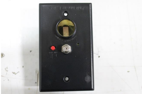
TV Signal Amplifier Power Switch (located next to the TV)
