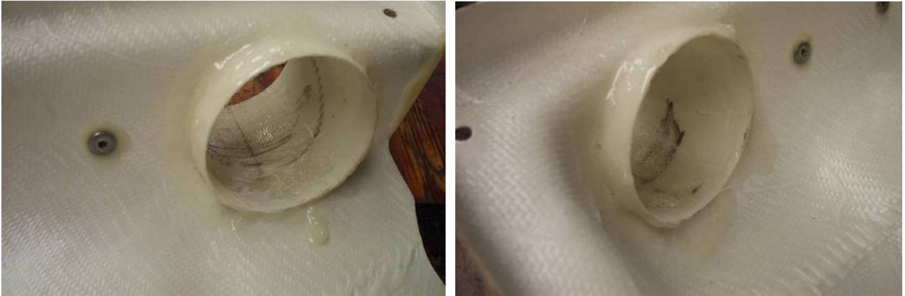
Figure 34. Air Filter Box Plumbing – Incorrect
