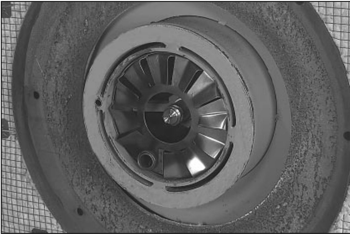
Standard CB Burner Housing (Rear View, Inside Front Head)
