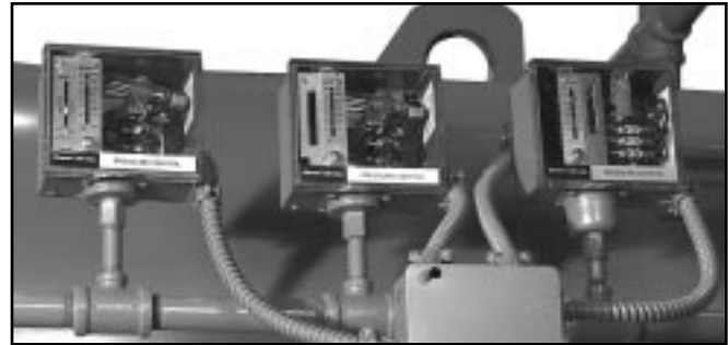
Figure: 6-7 Steam Operating Controls
