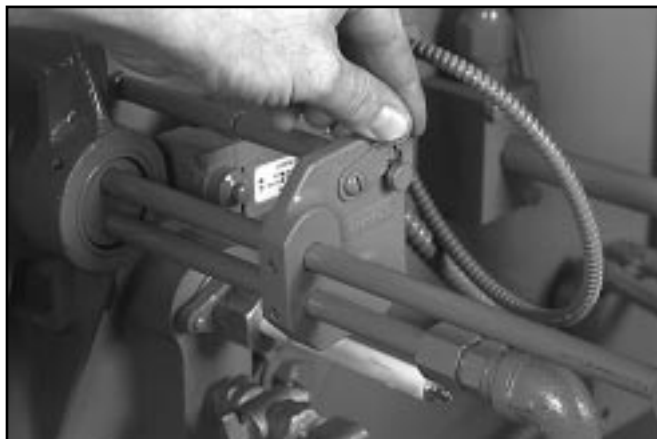
Figure: 5-13 Oil Gun Locked in OUT Position
