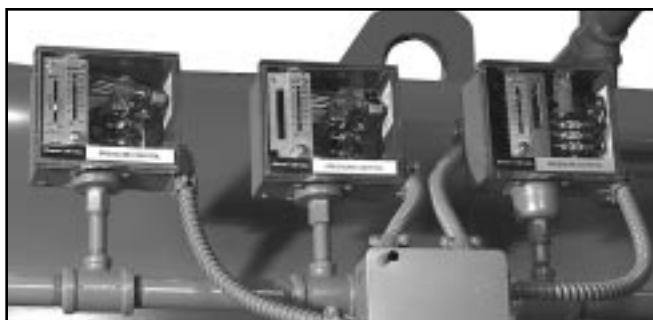
Figure: 6-4 Steam Operating Controls
