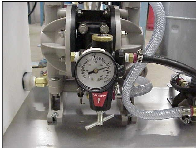
Pump Cart Pressure
