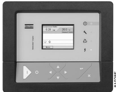
Control panel of the Elektronikon™ Graphic controller
